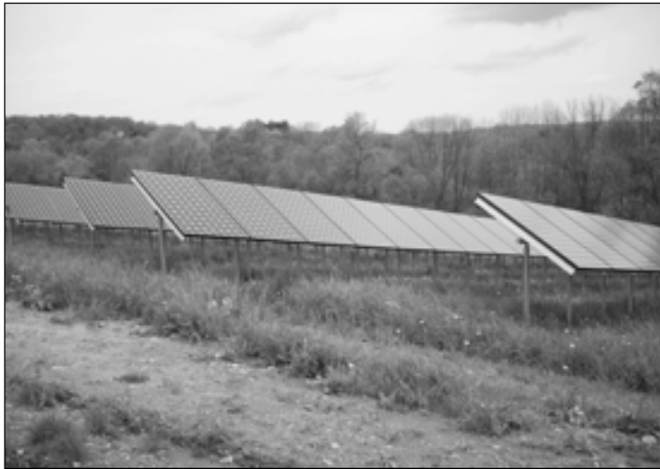
These solar panels stand along the eastern side of the Timex Group building. In all, 800 panels generate 285,439 kilowatt-hours of energy a year. (Cristina Commendatore photos)
